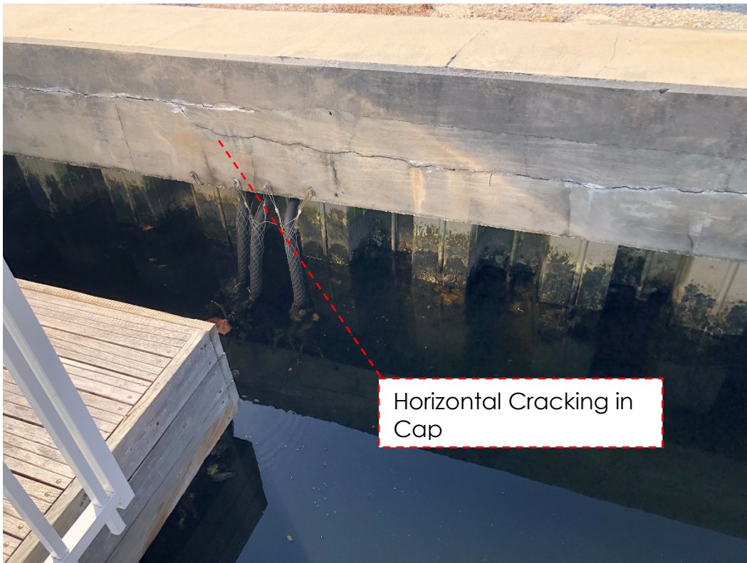
Photo #14 – View of Horizontal Cracking in Seawall Cap
