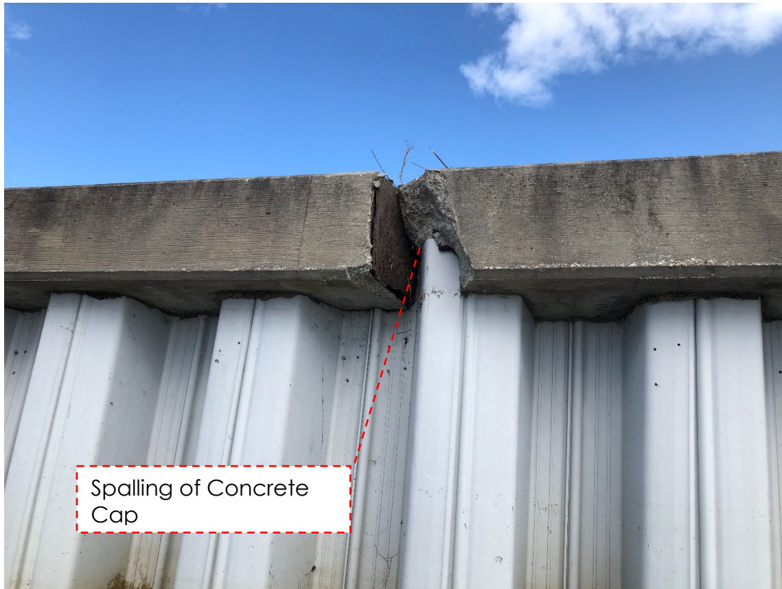
Photo #19 – Spalling Section of Seawall Cap at Expansion Joint
