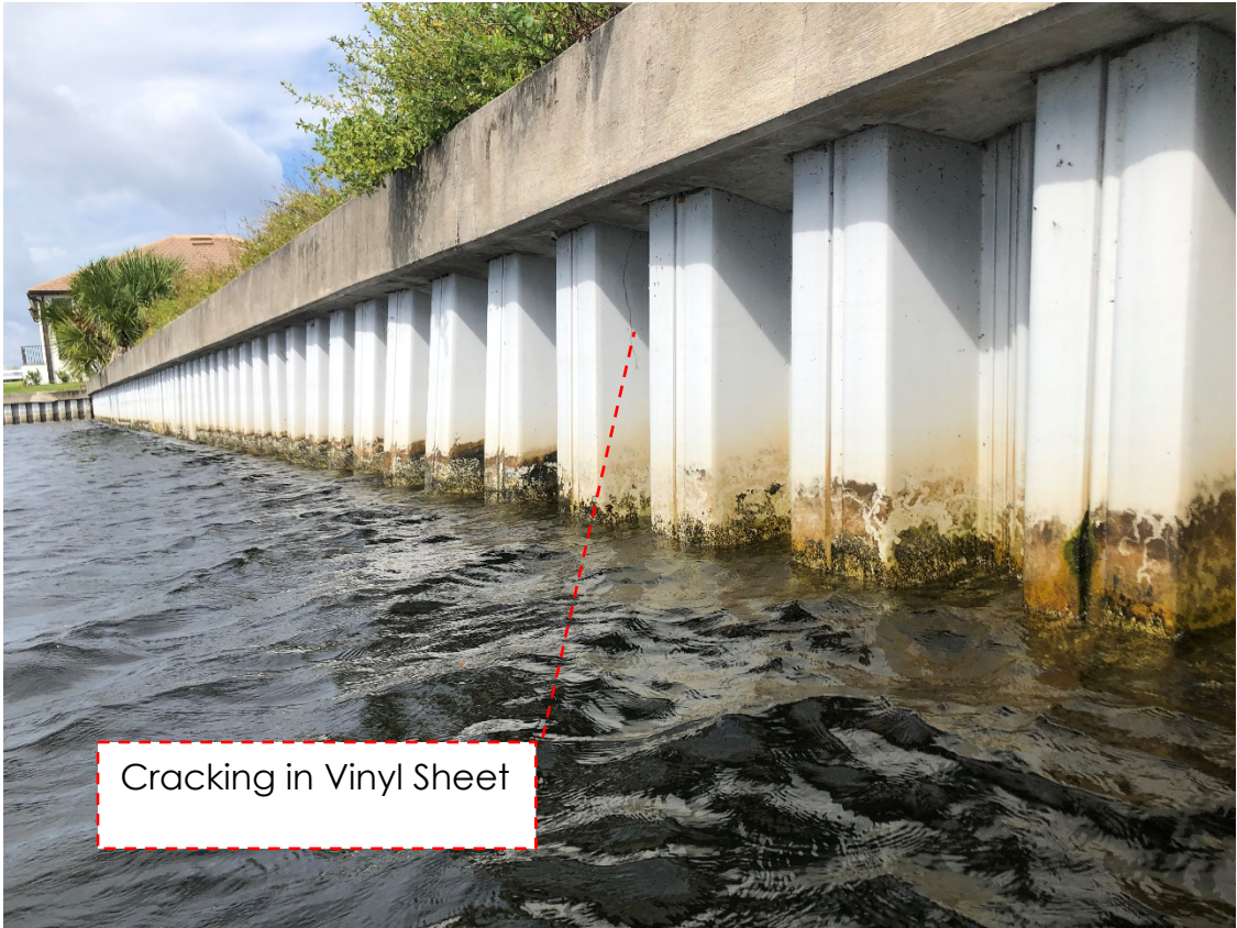
Photo #17 – Vertical Cracking at Top of Vinyl Sheet
