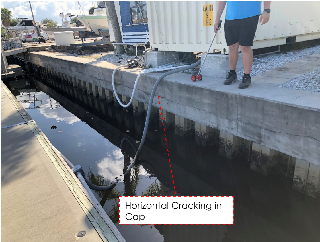
Photo #13 – View of Horizontal Cracking in Seawall Cap
